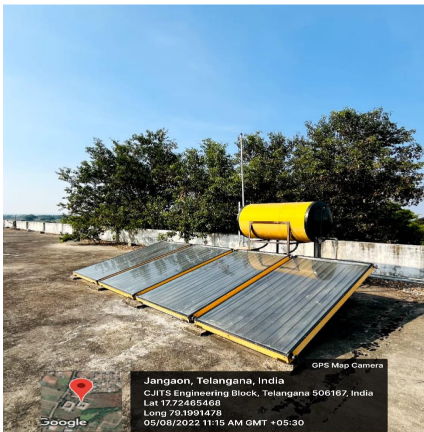
Fig1: Corner view of solar plant 10 Kwp
